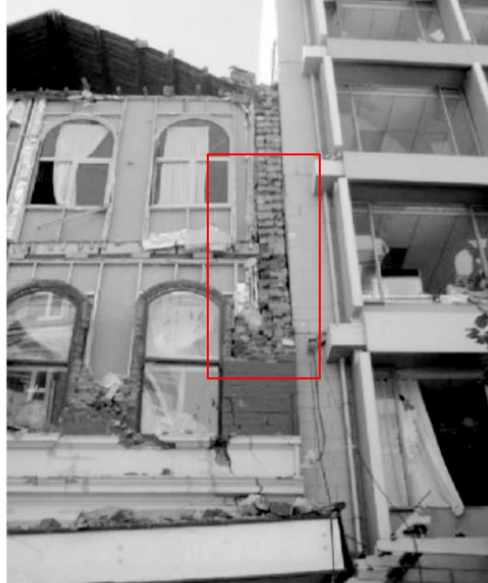
Figure 2.7. Pounding between unreinforced masonry and reinforced concrete buildings, adapted from (Cole et al., 2012)
