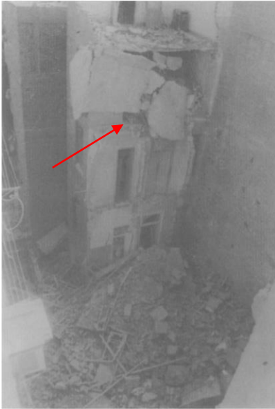
Figure 2.3. Failure of a load-bearing masonry house in Cairo adapted from (Badawi and Mourad, 1994)
