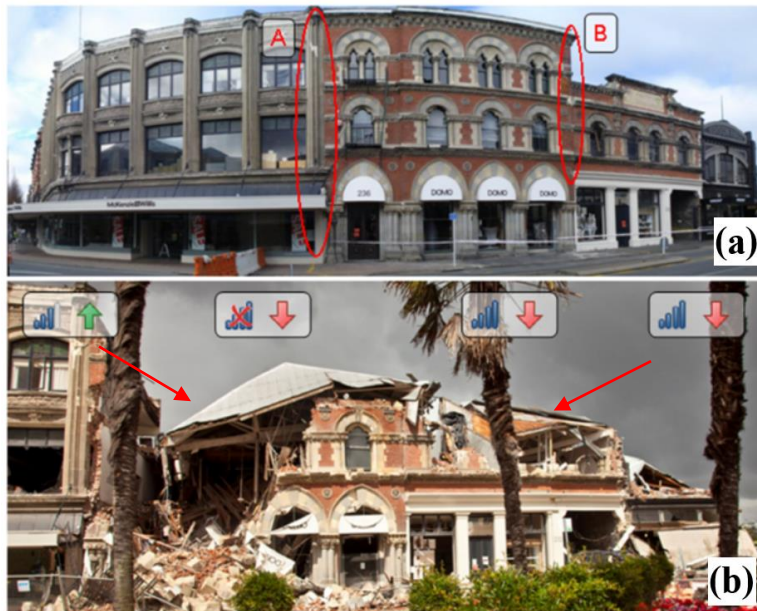
Figure 2.6. Pounding damage to masonry buildings: (a) damage after the Darfield event (panoramic image); and (b) damage after the Christchurch event, adapted from (Cole et al., 2012)
